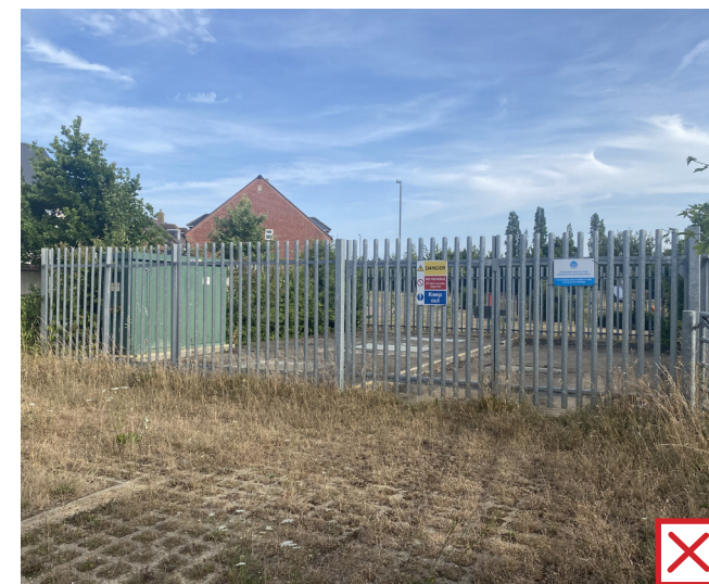
Water pumping stations not suitably screened by landscape
