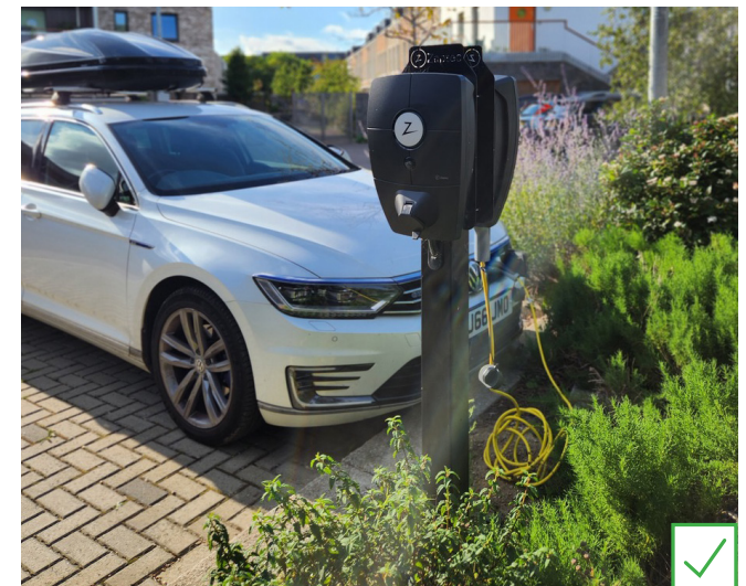
Example of a well-integrated electric vehicle charging point
